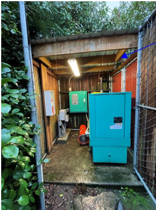
PS 1 – Generator Enclosure
