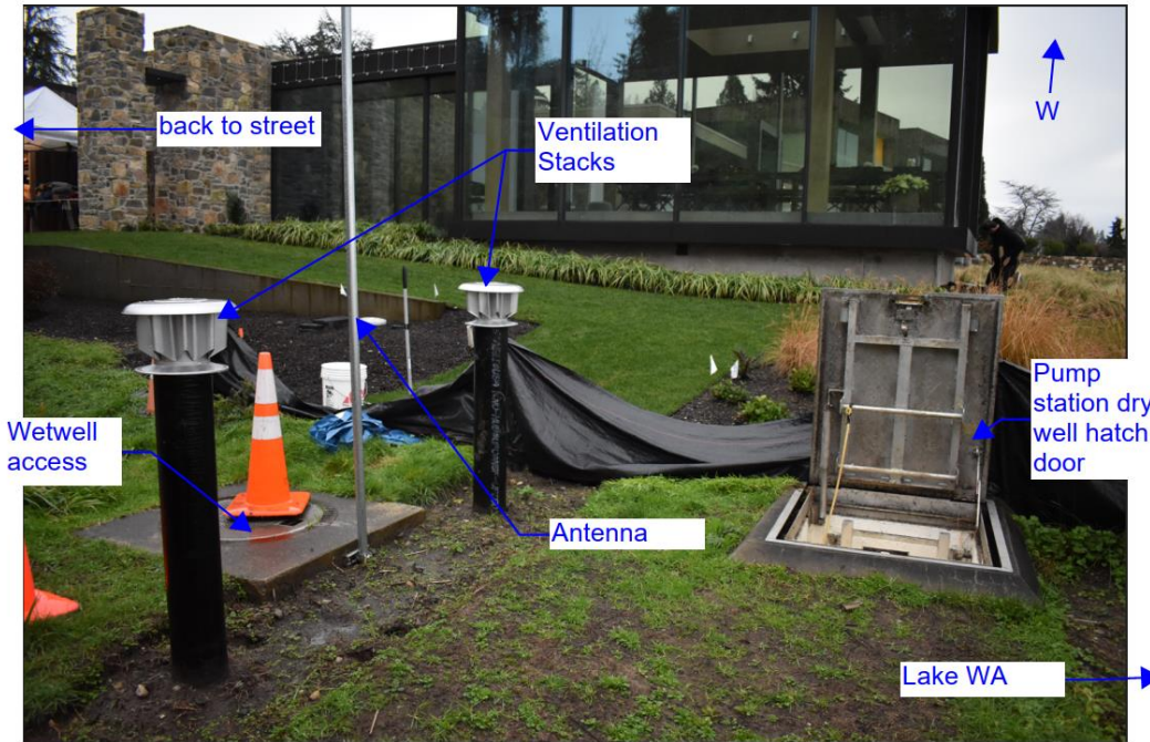
PS 1 – Pump Station
